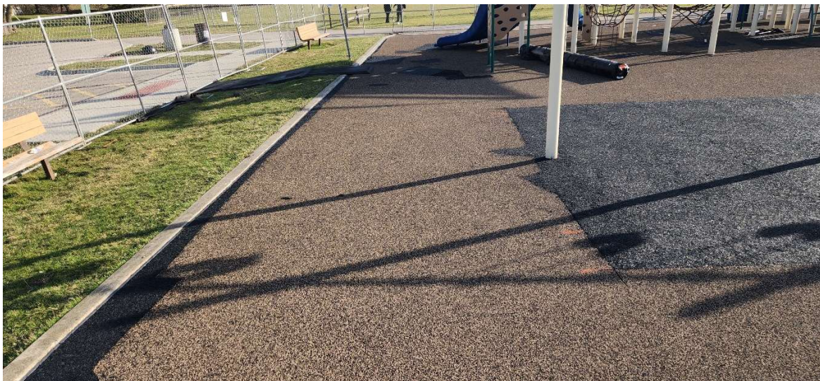
Edges were cut, nailer board installed, and sides infilled with new rubbering preparation for the turf.
