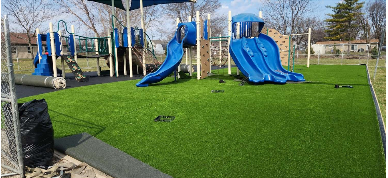
The artificial turf rolls are being laid out and cut around the posts
