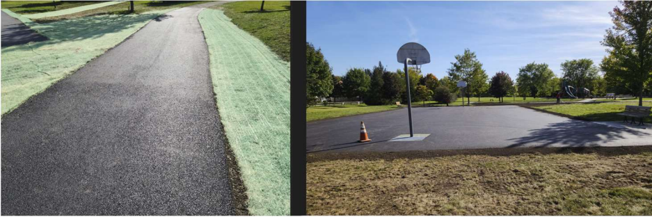
Sterling Meadows Park Basketball Court – New asphalt and landscape repair with seeding.
