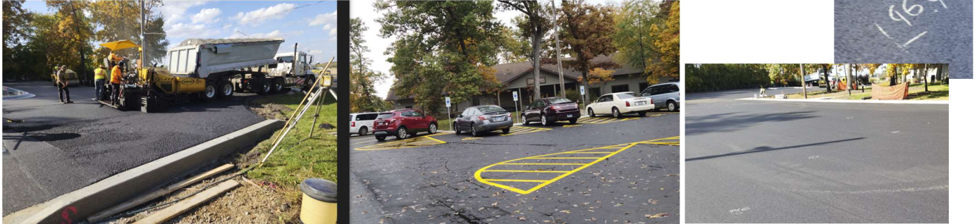
Grand Oaks Recreation Center – Asphalt installation, painted parking, testing for compaction density to breakage percentage – goal for testing numbers in the mid 90's.
