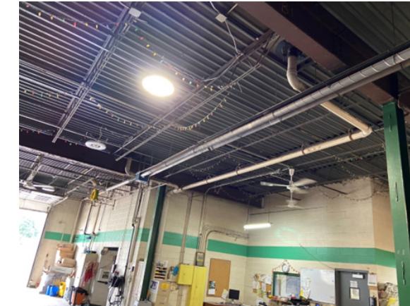
combination of newer LED and older fluorescent fixtures throughout facility
