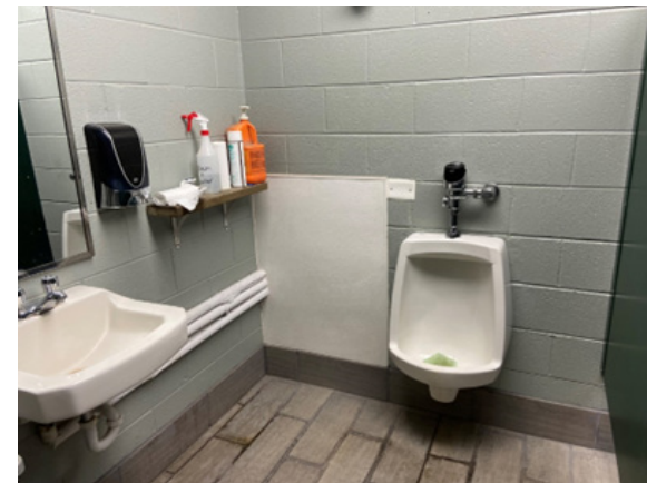
Degraded flooring in men's restroom
