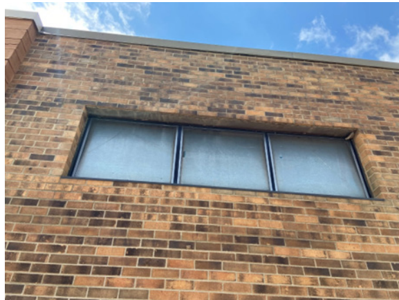
Existing windows and lintels (minor corrosion visible)
