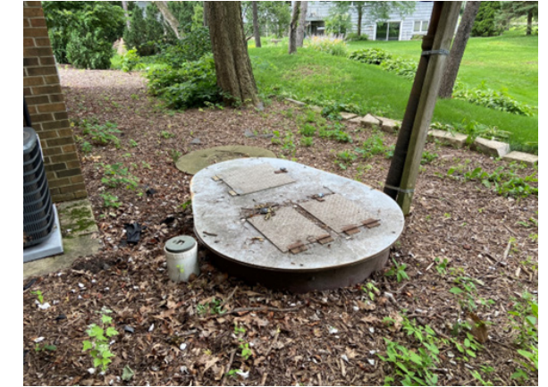
outgoing sanitary sewer cleanout / ejector
