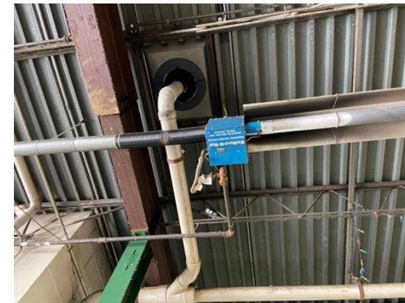
Infrared heating in main garage space
