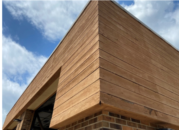
Minor damage/deterioration at wood siding
